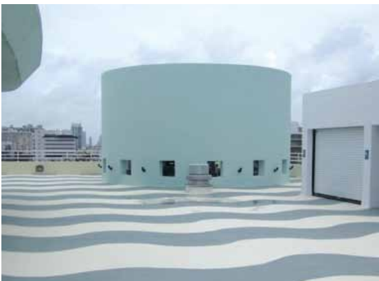
Cooling towers (enclosed in round structure)
