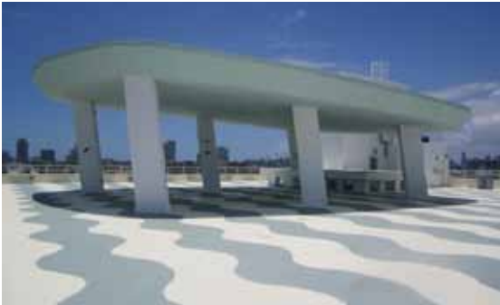
Rooftop area for outdoor events - safe for pedestrian use due to TrafficCoat's non-skid properties
